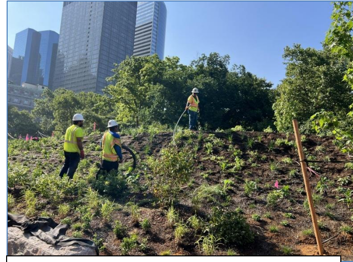
Battery landscaping installation
