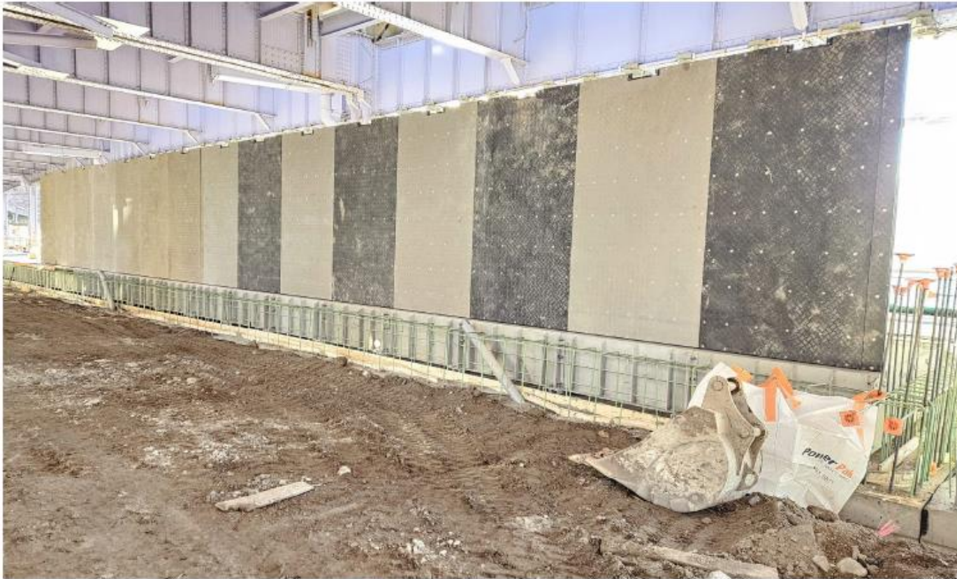
Flip up gate segments installed under FDR Drive near Robert F. Wagner Sr. Place – March 2026
